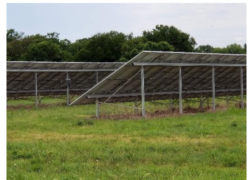
Example of a Solar Conversion System, Ground-mounted
