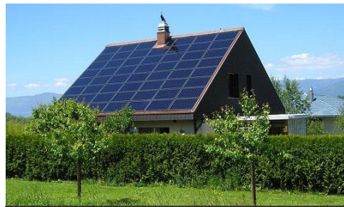
Example of a Solar Conversion System, Structure-mounted
